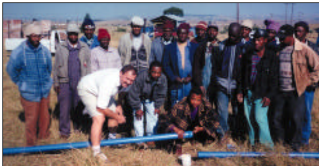
TANGA: DPI training persons from the local community (HDIs). Amanz'abantu supplied the pipes.
